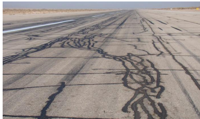
Figure 1. Overview of cracks in the Kerman Airport runway
