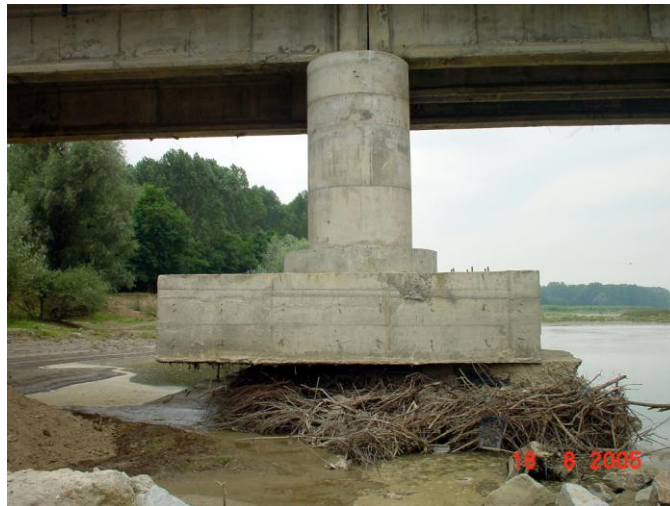
Photo 6. Modification of the hydraulic regime of the water channel (bridge over Siret River, at Ion Creangă, Bacău County – Romania)
