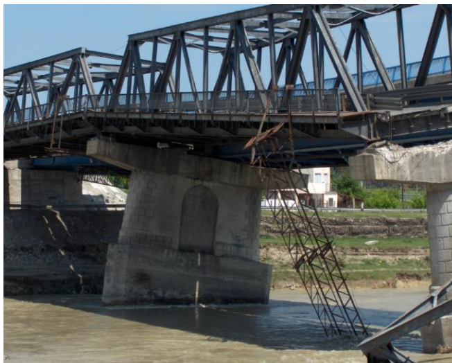
Photo 8. Damage of the superstructure due to infrastructure failure; bridge over Buzău River at Mărăcineni (Romania)
