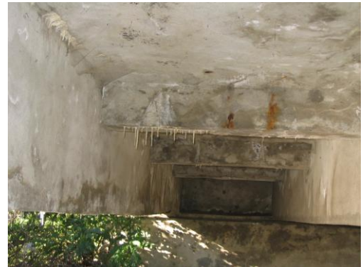
Photo 4. Infiltration, humid spots, stalactites (bridge over Sovata River, at Sacadat de Jos, Mureş County – Romania)
