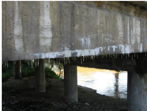
Photo 3. Stalactites (bridge over Bârsa River, at Ghimbav, Braşov County – Romania)
