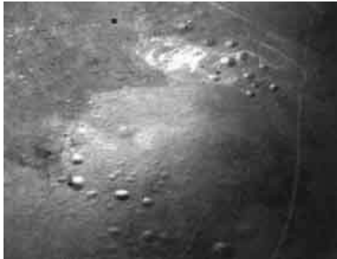
Figure 1: Separation of flooring from the base and creation of bulges
