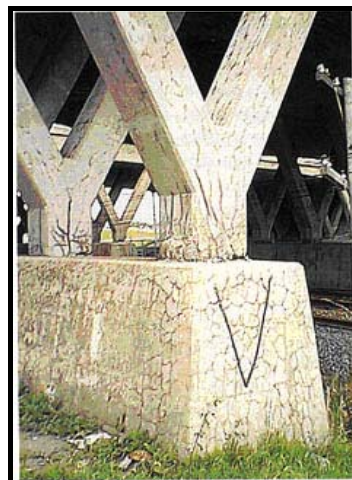
Figure 9. Network cracking (Source: http://www.filer.case.edu )
