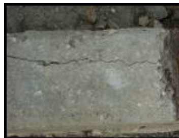
Figure 6. Corrosion crack (Source: http://www.upload.wikimedia.org )
