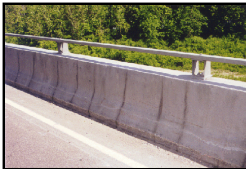
Figure 13. Temperature cracks (Source: http://www.irc.nrc-cnrc.gc.ca )
