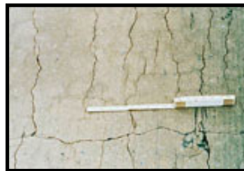
Figure 7. Alkali-aggregate reactivity cracks (Source: http://www.cement.org )
