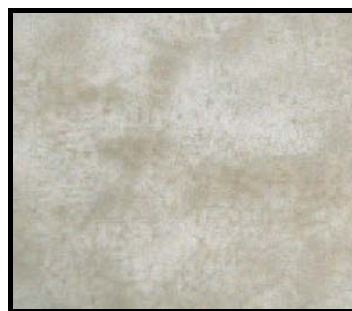
Figure 1. Craze cracks (Source: http://www.concreteconstruction.net )
