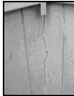
Figure 14. Shrinkage cracks (Source: http://www.inspect-ny.com )
