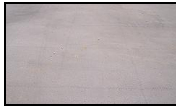
Figure 5. Drying shrinkage cracking (Source: http://www.members.optusnet.com.au )
