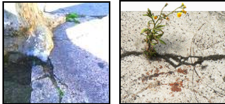
Figure 16. Environmental cracks (Source: http://www.ewhow.com ; http://www.imagination.lancaster.ac.uk )
