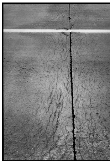
Figure 2. D-cracking (Source: http://www.concrete.org )
