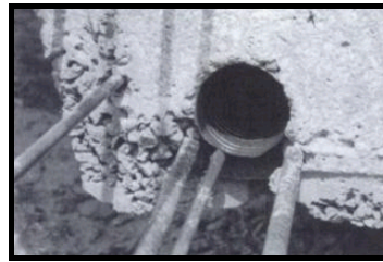
Figure 8. Honeycomb cracking (Source: Handbook of concrete bridge management De Jorge de Brito)
