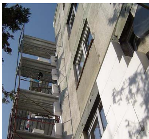
Figure 5. Building from Cluj- Napoca town in the process of rehabilitation with 15 cm of polystyrene EPS
