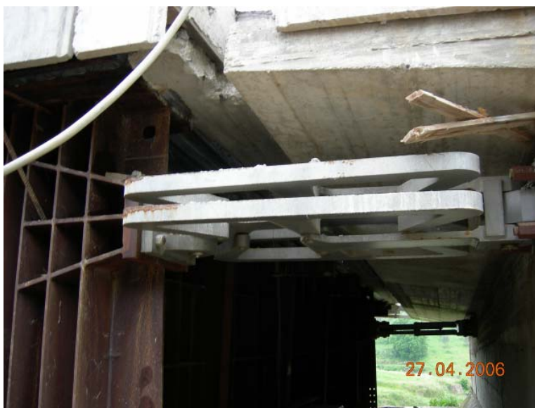
Figure 17. Application example of seismic isolation of existing viaducts by decks substitution and deployment of elastic-plastic dissipators on abutments
