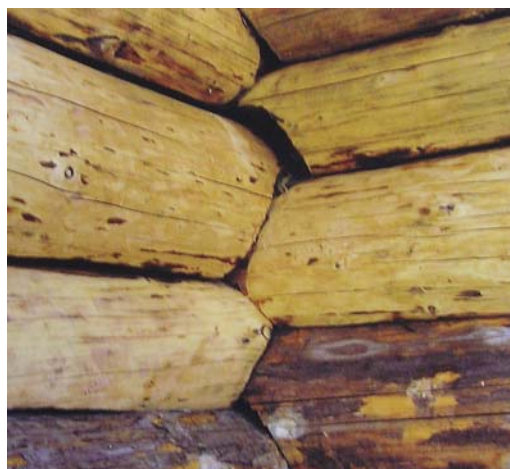
Figure 2. Incorrect corner structure (roughly encircled shapes)
