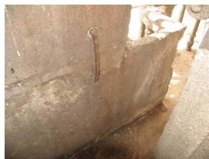
Figure 6. Left battlement of the facade
