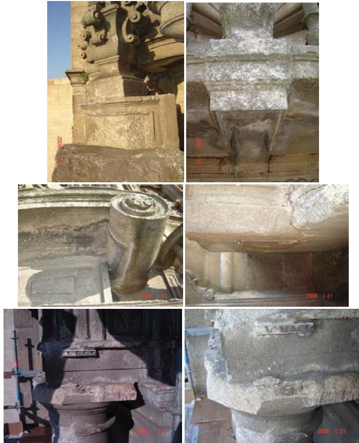
Figure 3. Deterioration of the granite – details in the slab, pinnacles and columns
