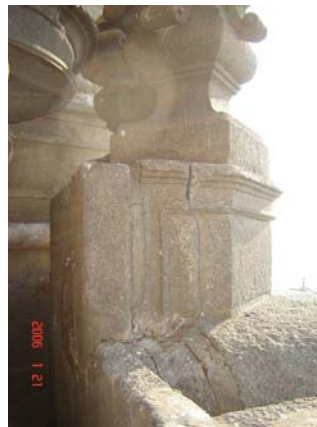
Figure 4. Detail of the detaching of pinnacles' structure from the battlement and view of the iron dowels on the back of the elements connecting the granite ashlars
