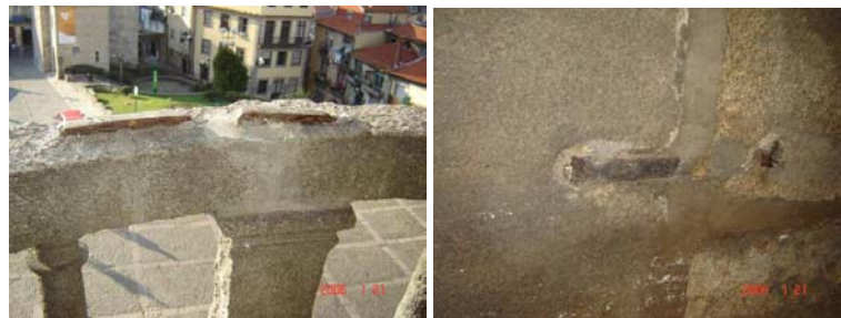
Figure 2. Details of the connection of the stones in the balcony's balustrade and between the ashlars of the slab
