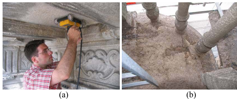
Figure 5. Central balcony: (a) inferior ribs of the slab, (b) steel connectors in the balcony's slab
