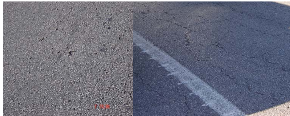
Figure 3. Distresses on EN 206 VARIANT: a) ravelling; b) cracking
