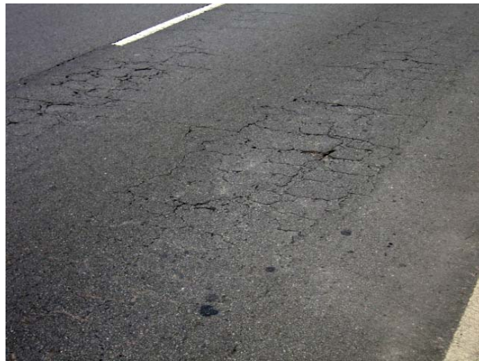
Photograph 2 – Pavement in failure condition
