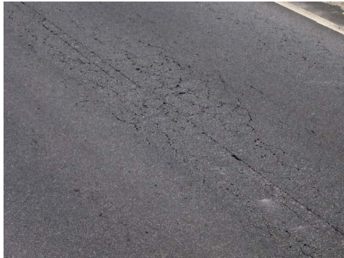
Photograph 1 – Cracked pavement (alligator cracking): pre-failure condition
