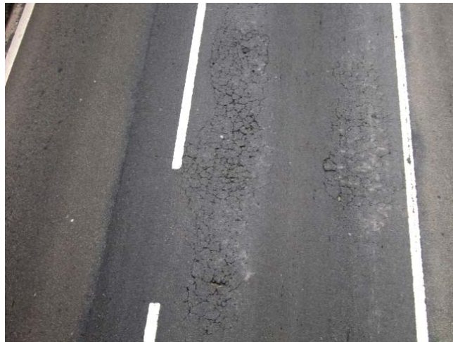
Photograph 4 – Deteriorated pavement of a high traffic capacity urban road
