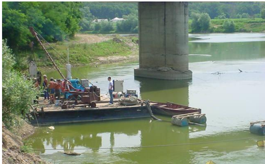
Fig. 8. Bridge over Siret river at Ion Creangă – consolidation and safety works at pier 10
