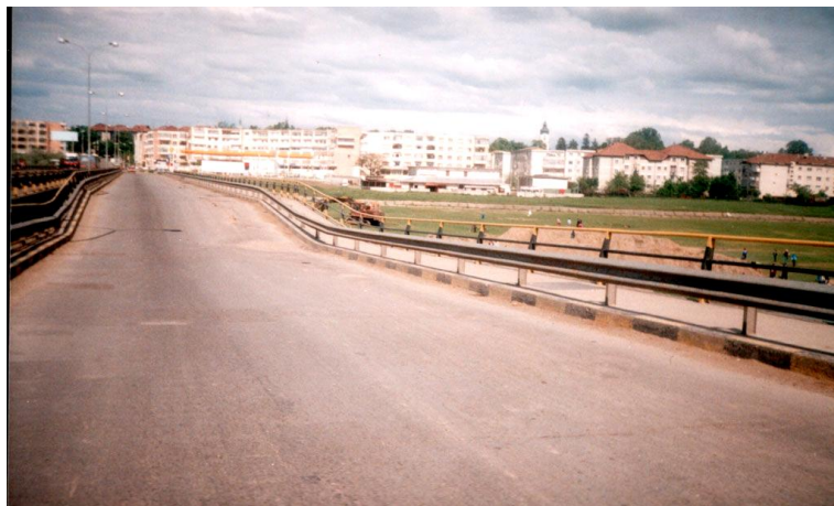
Fig. 2. View on the deck of the bridge over Moldova River, at Roman, after failure of pier nr.4
