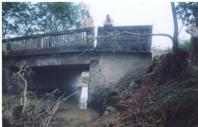
Fig. 4. Displacement of the abutment from the initial position and destruction of wingwalls
