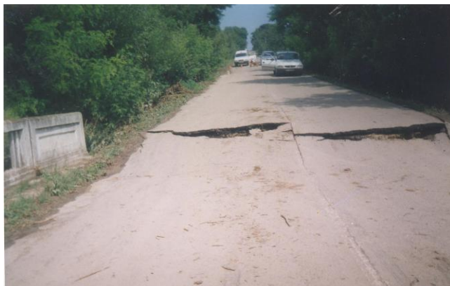
Fig. 5. Failure of backfill behind the abutment
