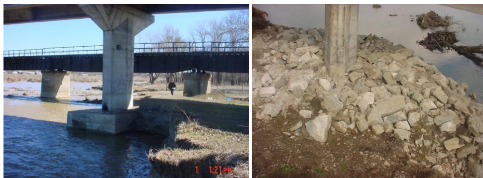
Fig. 7. Bridge at Dornești: displacement of the channel toward banks, before and after consolidation
